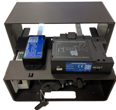
Small inspection grate – inside
